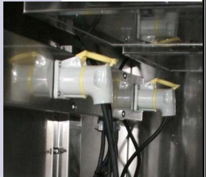
Illustration 2.D: Dual Serving Module Power Cord Plugged into Rear Distribution Panel of Flex Serving Line Cabinet
