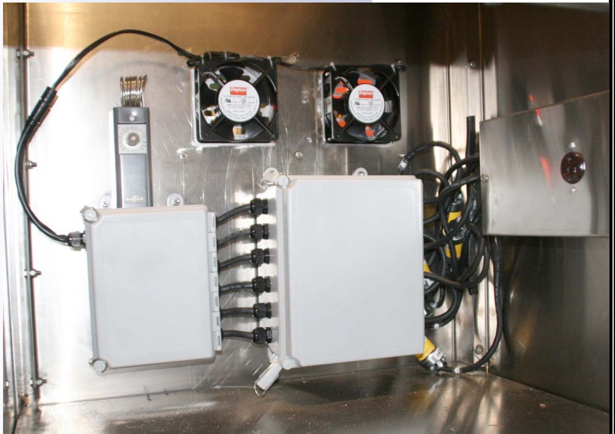
Illustration 2.B- Breaker Box, Distribution Block Box, Rear Distribution Panel
