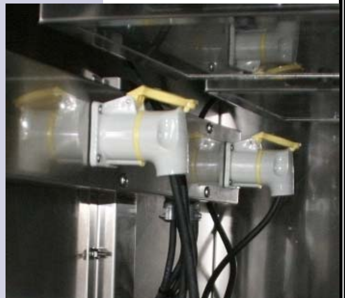
Illustration 2.D: Dual Serving Module Power Cord Plugged into Rear Distribution Panel of Flex Serving Line Cabinet
